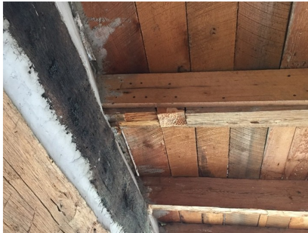
Charred log near ceiling of Higgins House
